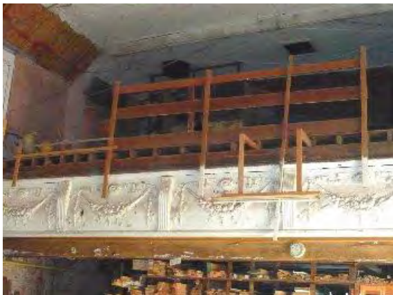
The old Pavillion Theatre's balcony decoration. The projector room was at the rear.
